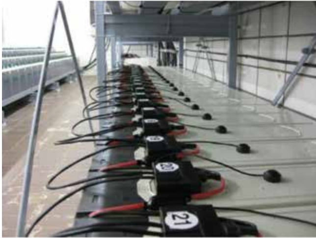
Civil Aviation Authority Installation, Europe
