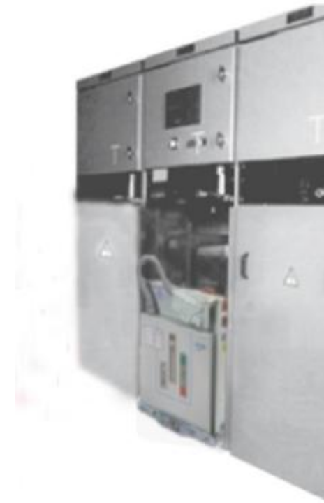
AFTER (Door Abandoned)
